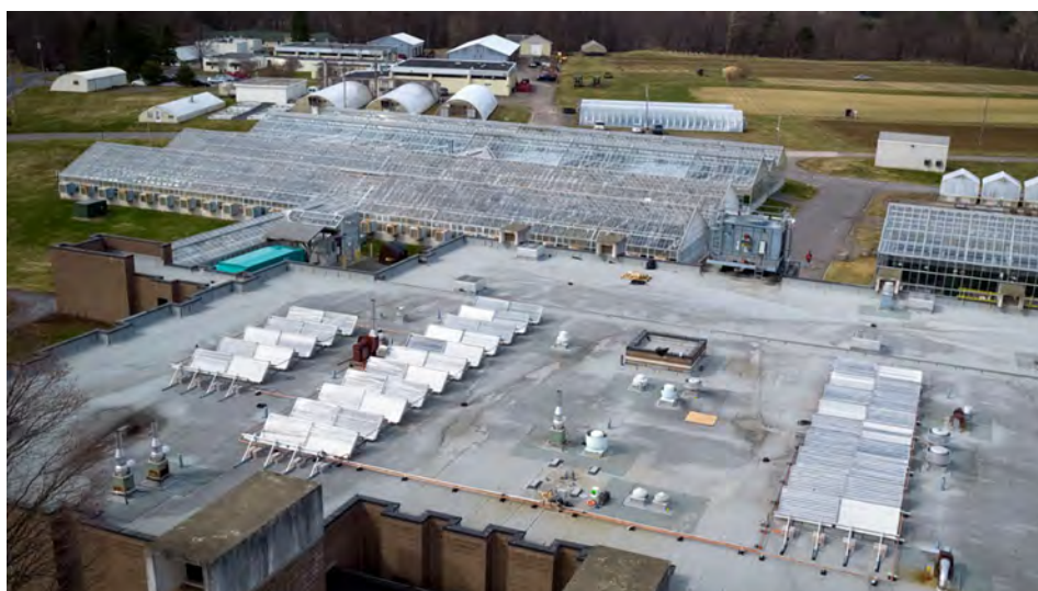
A new solar collector system installed atop Guterman Research Center uses innovative mirror technology to capture sunlight and turn it into thermal energy that will help heat the facility's water distribution network. (Lindsay France/Cornell University)
